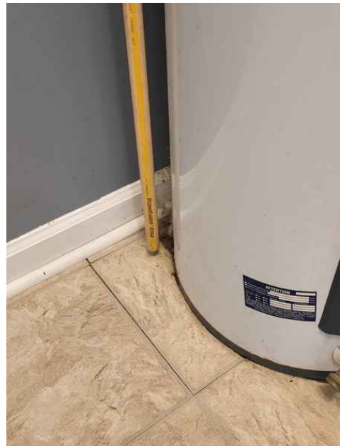
No Drip Pan at water heater
