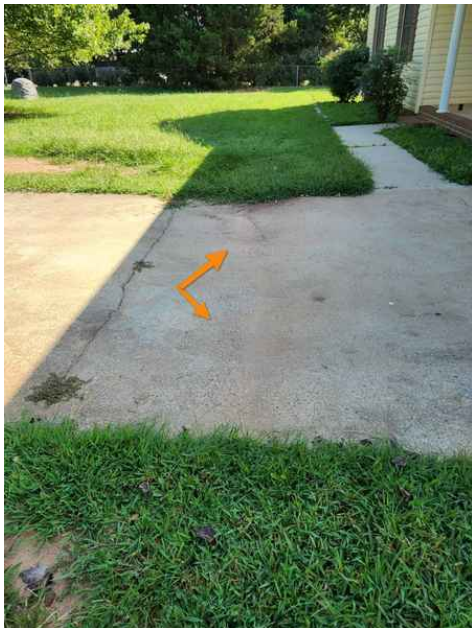
Low grade area of driveway
