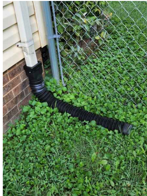
Correctly installed gutter downspouts that are diverting the water away from the foundation.
