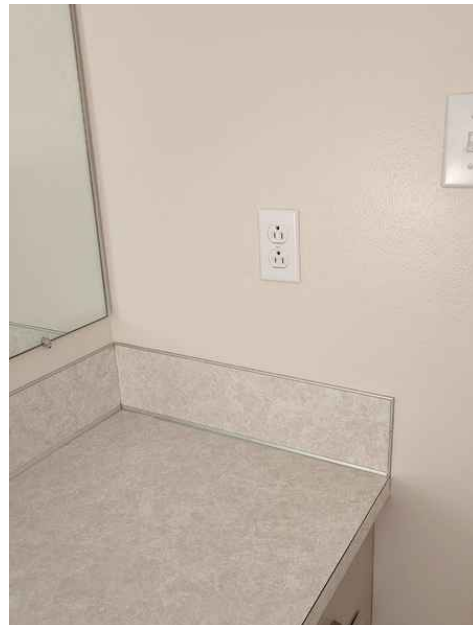
No GFCI protection on receptacle in master bathroom
