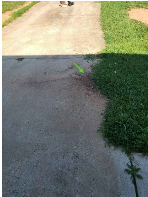
Area where water has pooled in low area of driveway
