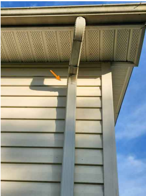
Downspout is missing strap near the eave which has allowed the downspout to move from its proper location.
