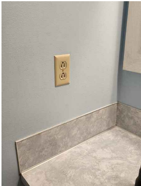
No GFCI protection on receptacle in hall bathroom
