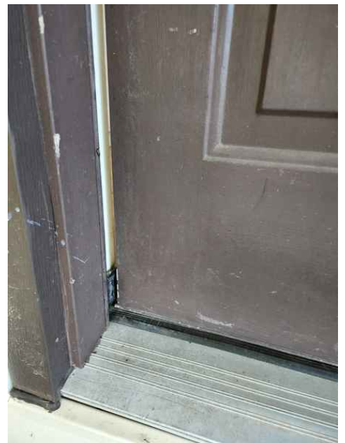
Door at carport sticks when opening or closing
